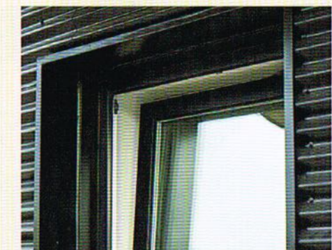
The triple-glazed windows allow for great insulation, but they're also easy to clean and good-looking. Straka used rigid foam on the outside of the house and spray-in foam inside to fill every gap.
